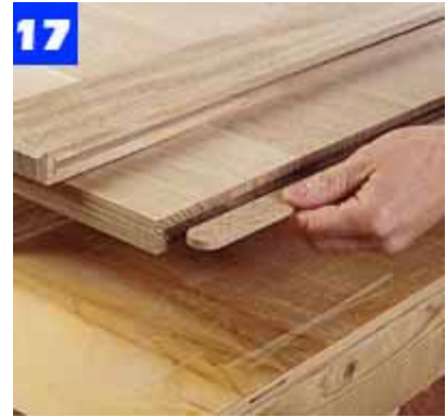
Cut splines for the breadboard-end joints. A 1/2-in. radius on the ends matches the slot profile.
